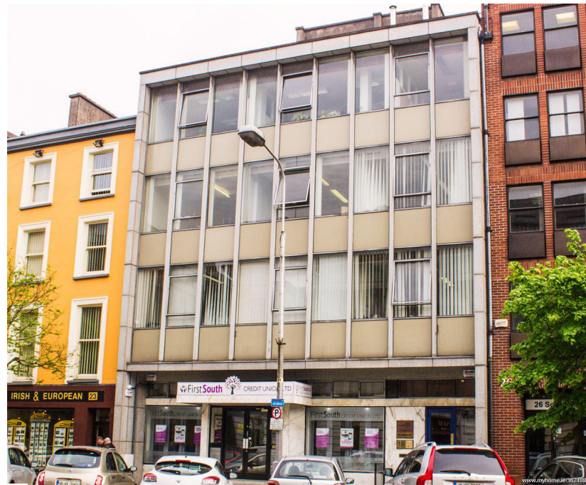
1 24/25 SOUTH MALL NORTH FACE FEATURES A STICK SYSTEM CURTAIN WALL. A GRANITE FRAME OUTLINES THE BUILDING WITH JOINTS MATCHING GRALZING PANELS HEIGHTS. GROUND FLOOR FEATURES A MARBLE FACADE AND TILE MOSAIC ON OVERHANGING AREA. SOUTH/EAST/WEST FACADES ARE A SAND CEMENT RENDERED FINISH.
