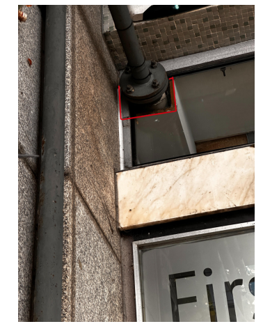
9 PENETRATIONS MADE INTO THE BUILDING. A LACK OF AIRTIGHTNESS MEASURES ARE VISIBLE.
