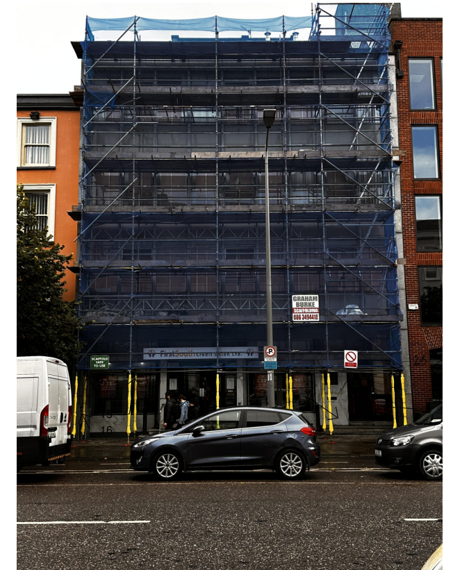
2 FRONT FACADE AS OF 06/10/23 COVERED IN SCAFFOLDING AND NETTING. UNKNOWN WORKS BEING CARRIED OUT.
